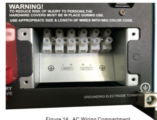
Figure 14 AC Wiring Compartment
